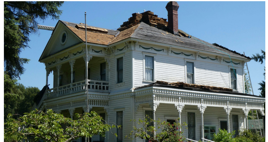
In the process of tearing off old shingles and installing new, cedar shingles, original skipjack boards were exposed on the east side of the Neely Mansion roof, 2023. Photo: Neely Mansion Association, Linda Van Nest
