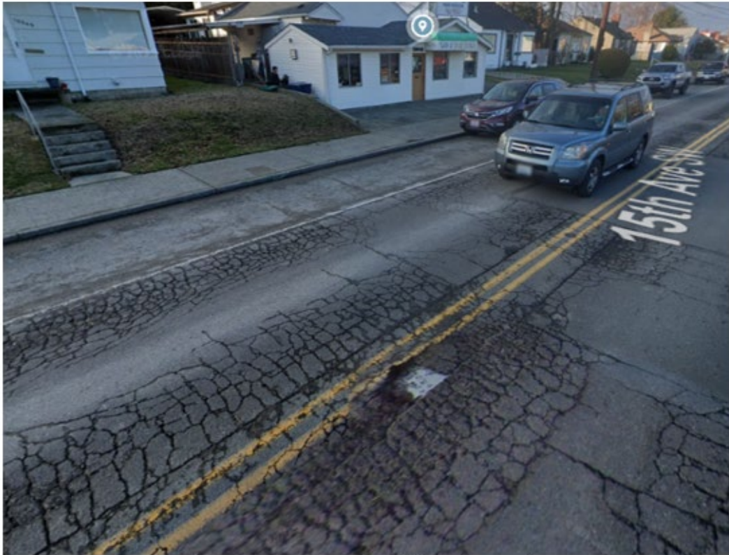
15th Avenue SW has a pavement condition is rated as a 0/100. This transit route in urban UKC was last paved in 1996.
